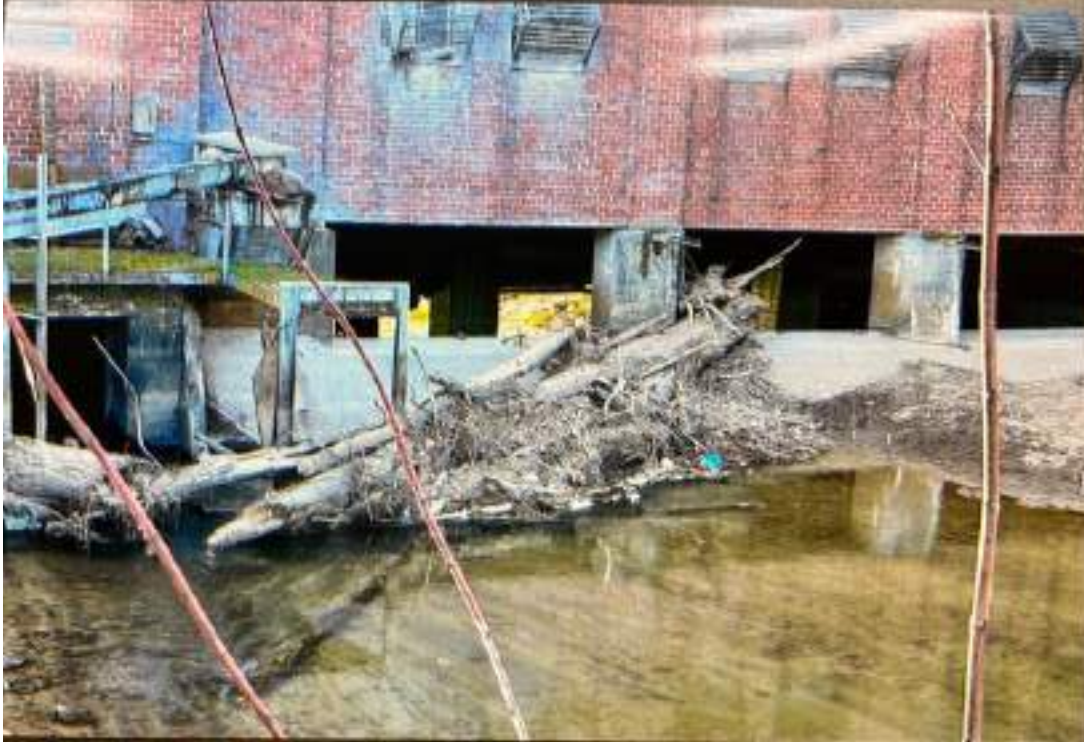
Figure 642: Debris Gathered on Upstream Side of Abandoned Mill Building in North Tazewell
