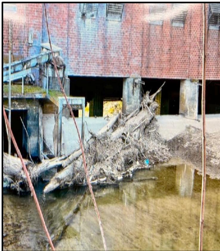
Figure 2. Debris Gathered on Upstream Side of Abandoned Mill Building in the Town of Tazewell
