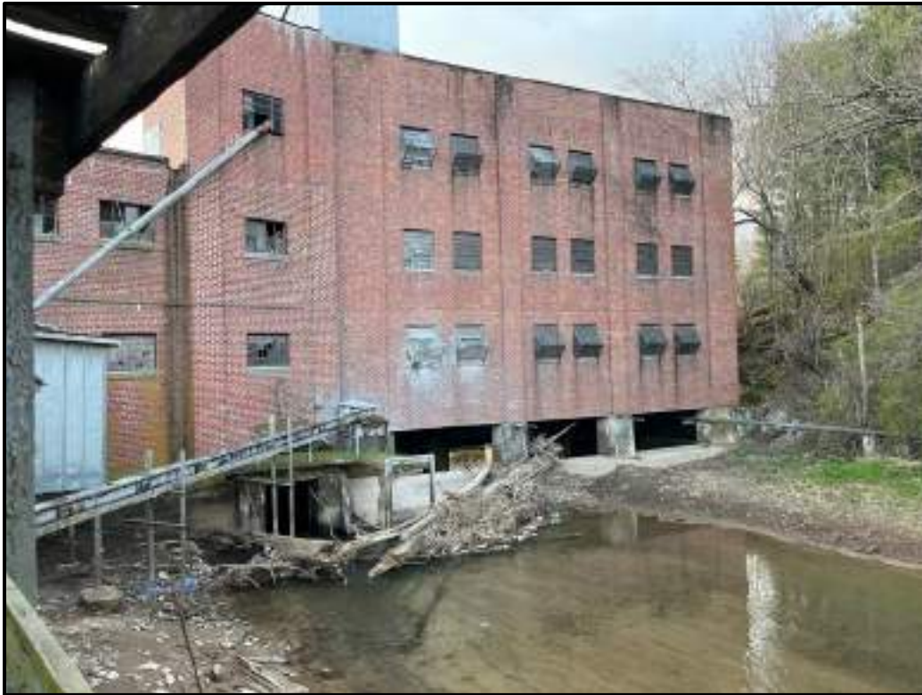
Figure 71: Mill Building March 2023 capturing debris
