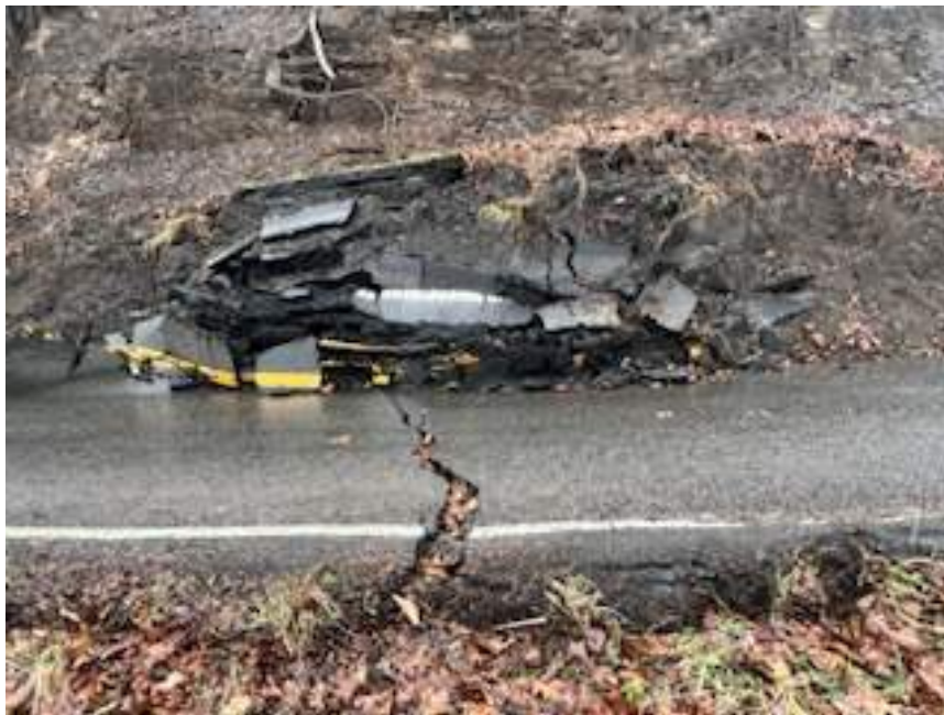
Figure 647: Damage from Landslide Event on Route 91
