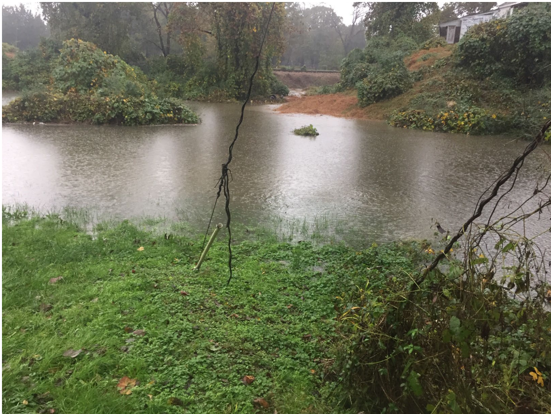
Overbank Flooding of open channel drainage system in the area downstream of Finney Outfall in a rain event on November 12, 2020. Photo is looking downstream towards CSX Railroad, the Suffolk Seaboard Coastline Trail, and the historic Cedar Hill Cemetery. This event also related in flooded utility infrastructure.
