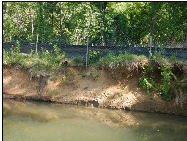
Highly eroded bank along Tuscarora Creek.
