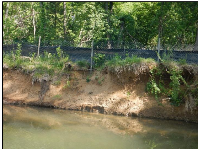
Highly eroded bank along Tuscarora Creek.
