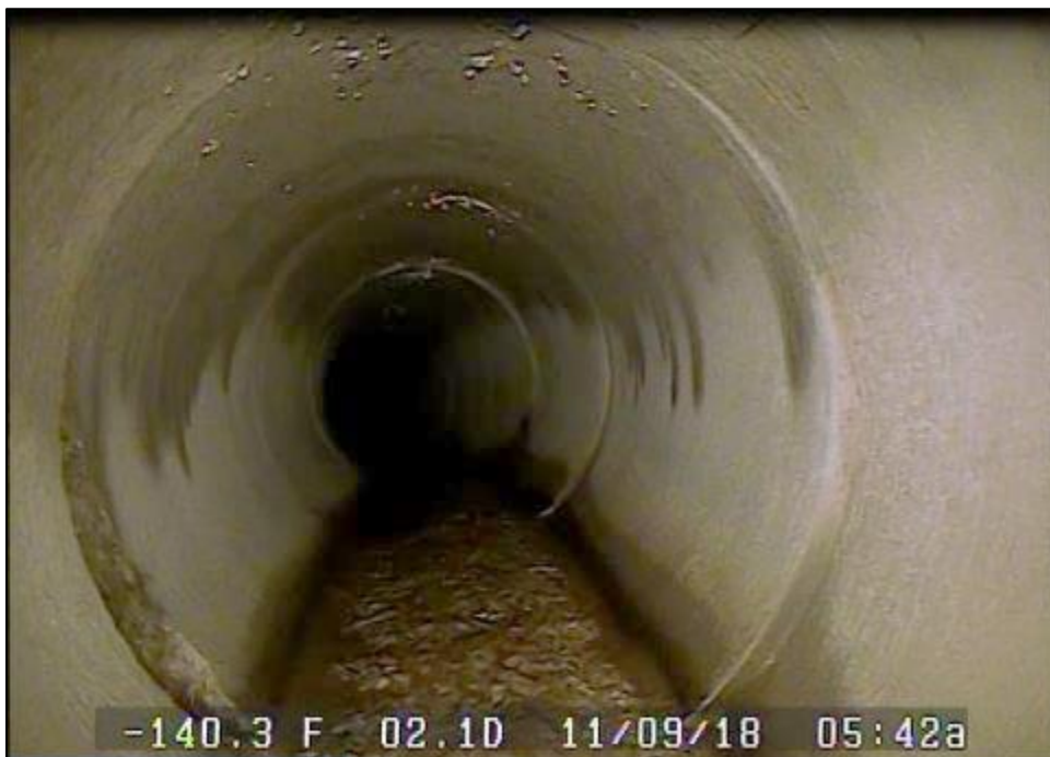
24" RCP Located Beneath Mickey's Body Shop Building
