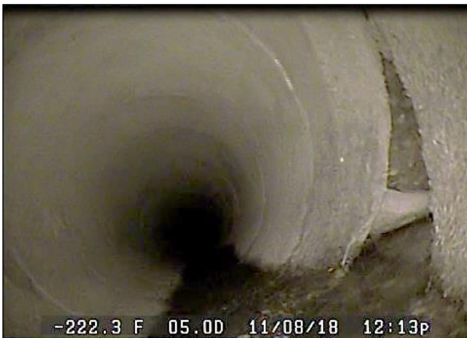
Defect in 36" RCP Pipe Beneath Guynn Furniture Building
