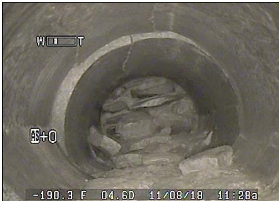
Plugged End of Abandoned 36" RCP at Swanson Street
