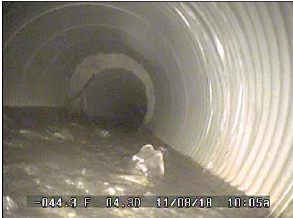
Pipe Constriction from 42" CMP to 36" CMP at Swanson Street
