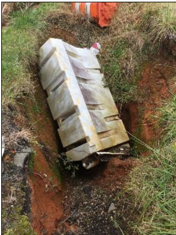
Sinkholes in Alley Between Lafayette and Monroe
