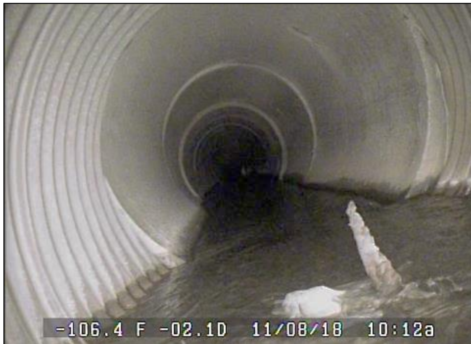
Pipe Transition from 36" CMP to 36" RCP at Swanson Street
