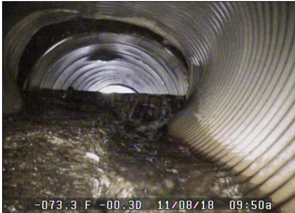
Pipe Blockage Near Swanson/McArthur Intersection
