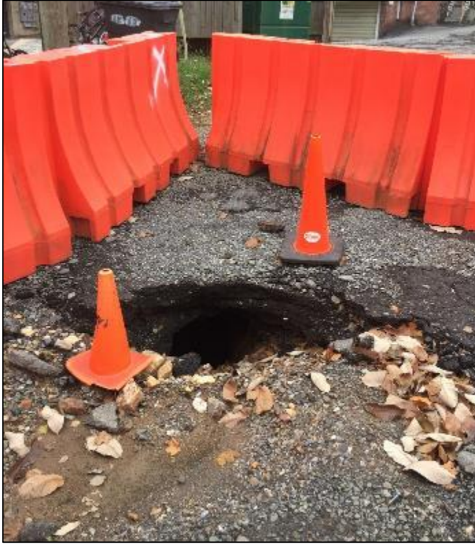
Sinkhole in Alley Near Madison Street
