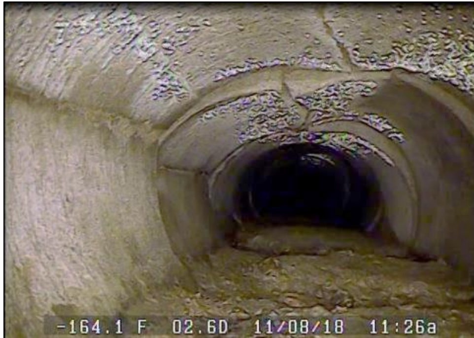
Deformed Interior of Abandoned 36" Pipe at Swanson Street
