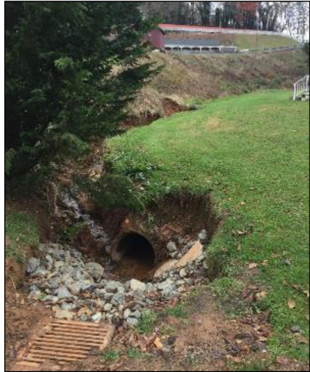
Erosion Around Blocked 30" Pipe
