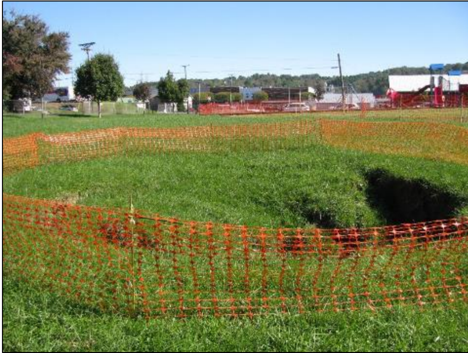
Pipe Collapse Location in Galax Elementary Playground
