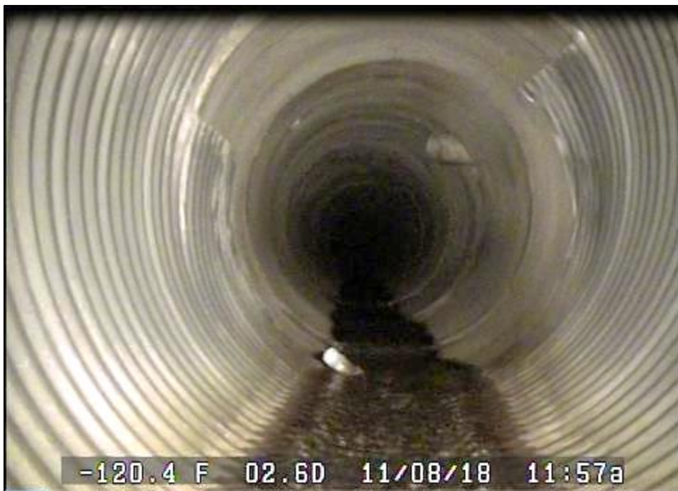
Transition from 42" CMP to 42" RCP
