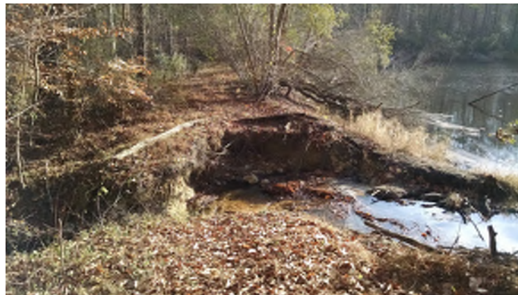
Image 2: Damage to Ennis Pond Earthen Dam after Hurricane Matthew (2016)
