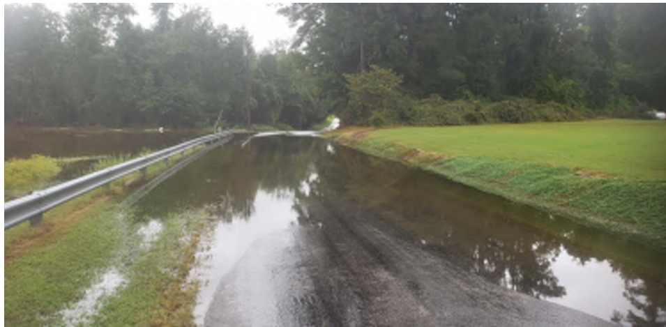
Image 1: Flooding on Woodland Drive in Isle of Wight County (September 9, 2020)
