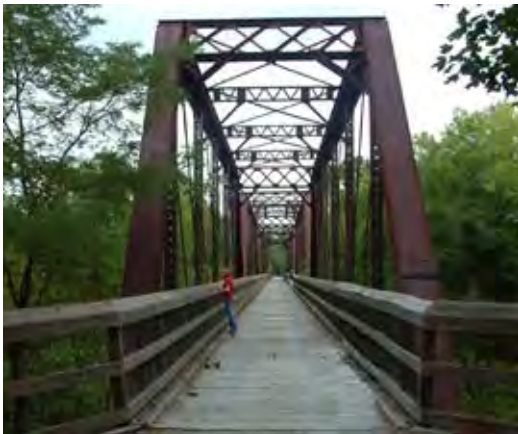
Rehabilitated bridge at Staunton River Battlefield State Park. Courtesy of LPDA, Inc.
