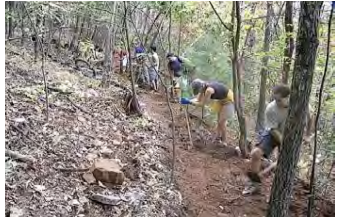
Selectively thinning vegetation to make room for a trail. Courtesy of IMBA/Rich Edwards.
