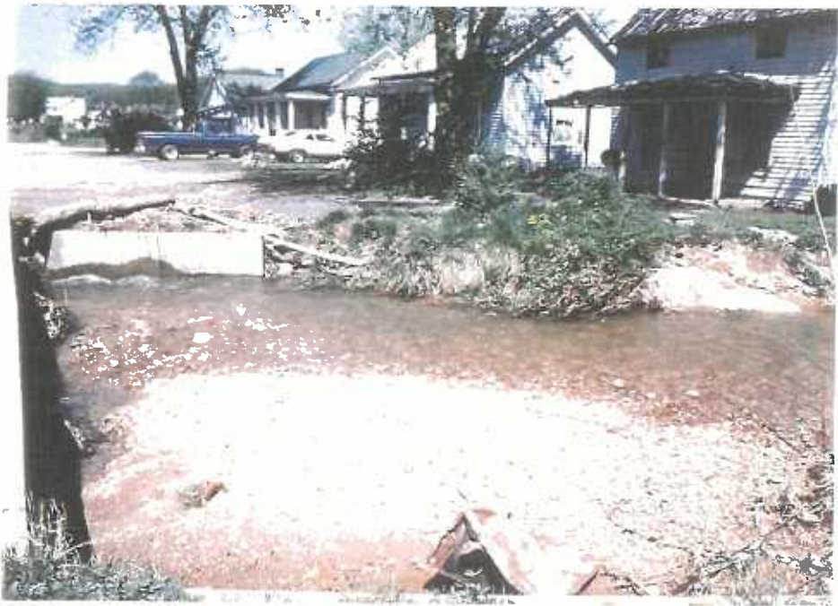
Sediment and debris blocking street culvert on Noels Run after April 1992 flooding.
