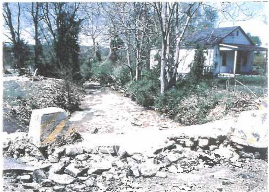
Destruction of street and blockage of street culvert with debris and sediment on Pedlar Gap Run from April 1992 flood.
