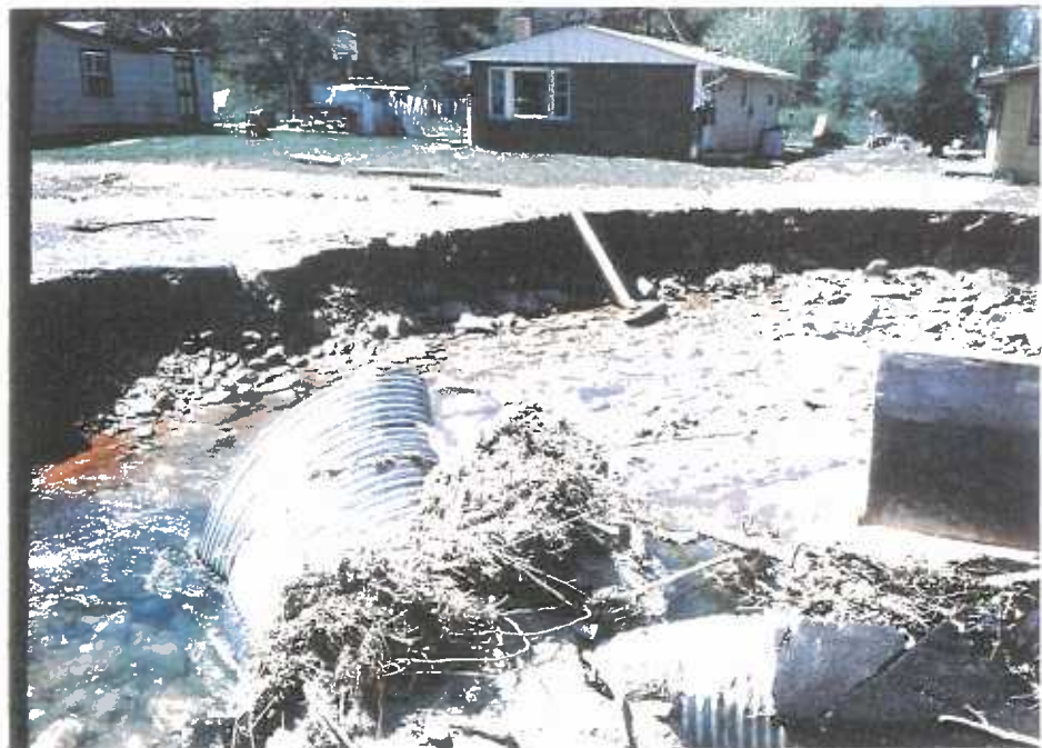
Destruction of culvert on Hawthorne Avenue from April 1992 flood.
