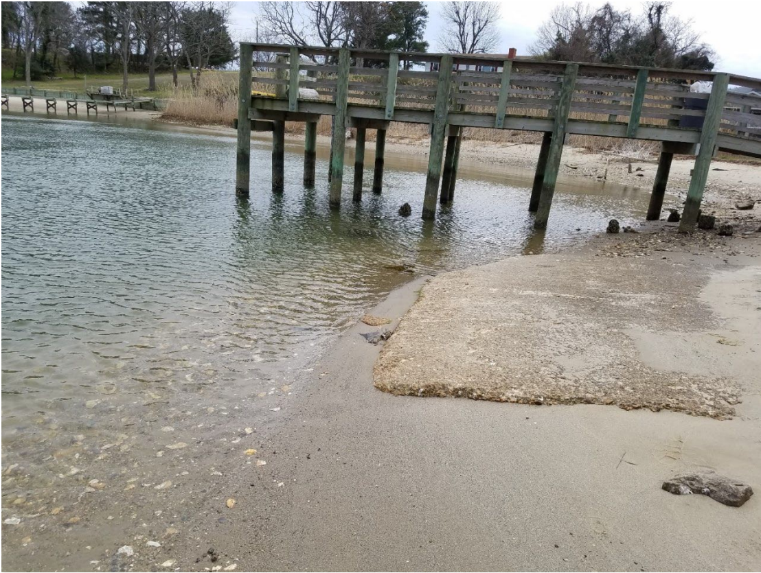
Whiting Creek Boat Ramp to be targeted for improvement in the proposed beneficial reuse design.
