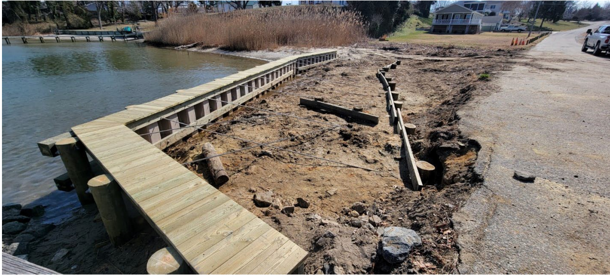
Shoreline protection improvements, initiated after the Jan. 4, 2022, opening of CFPF Round 3; photo taken March 1, 2022
