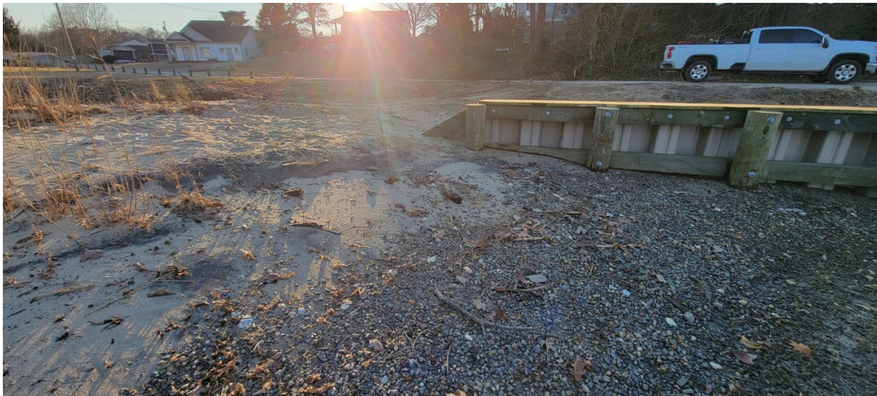
Shoreline protection improvements, initiated after the Jan. 4, 2022 opening of CFPF Round 3; photo taken March 1, 2022
