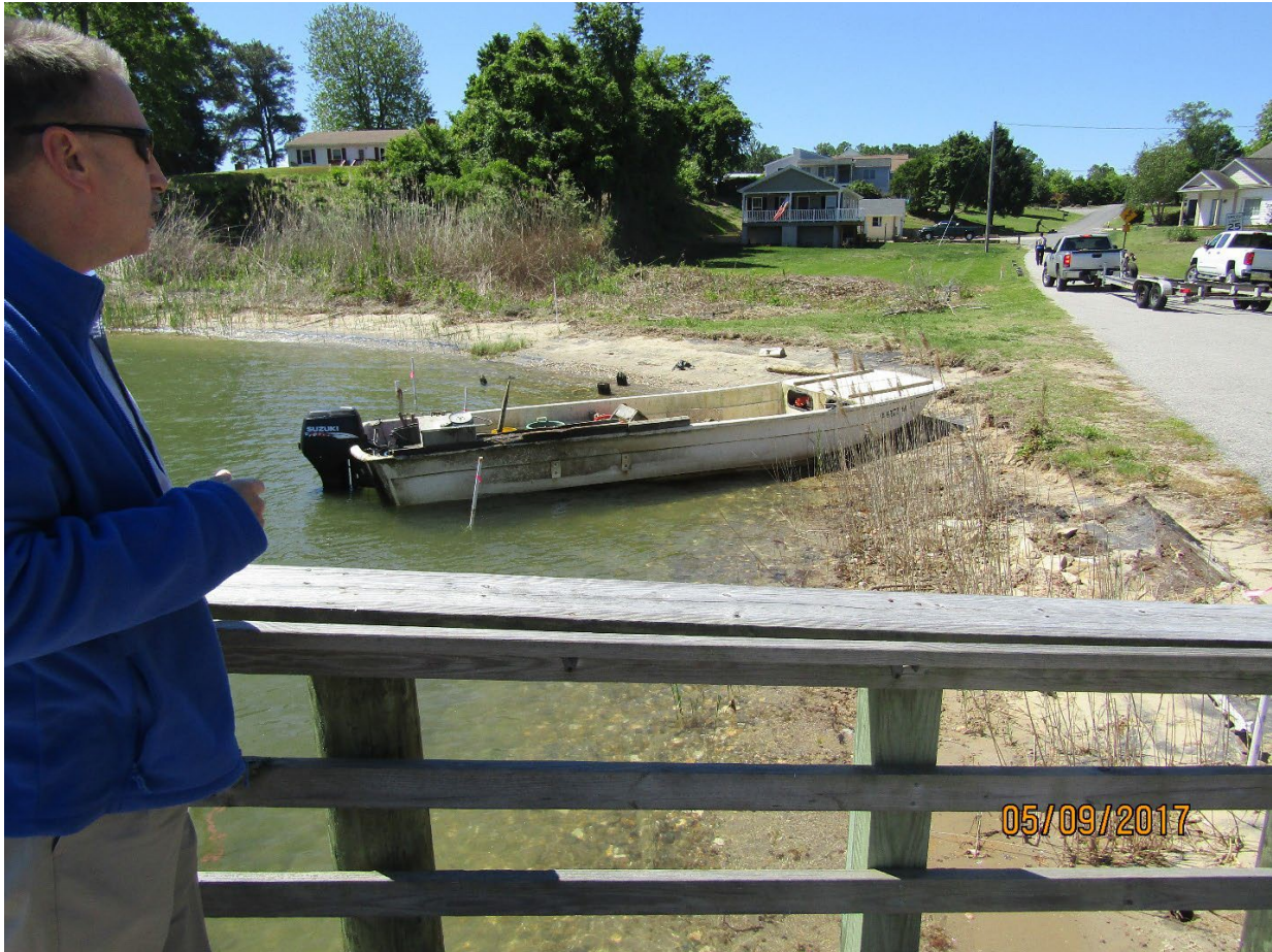
Eroded shoreline at project site from fishing pier prior to improvements. Note commercial fishing boat and active use by recreational and commercial boaters.
