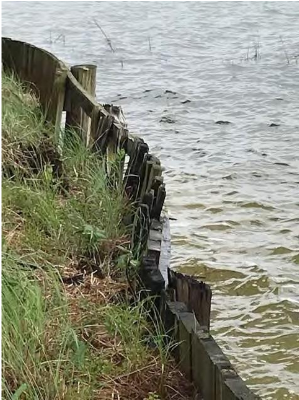
Photo of failing bulkhead.
