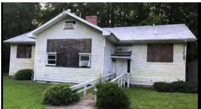
Photograph showing the current exterior front of the Historic Antioch Rosenwald School building. The current asphalt shingled roof is failing and is proposed to be replaced with a vegetated green roof or other stormwater collection roofing system.
