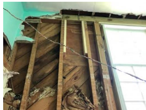
Photograph showing recent stormwater-related damages to the Antioch Rosenwald School building interior. Immediate assistance is needed to prevent further damages from the failing roof.
