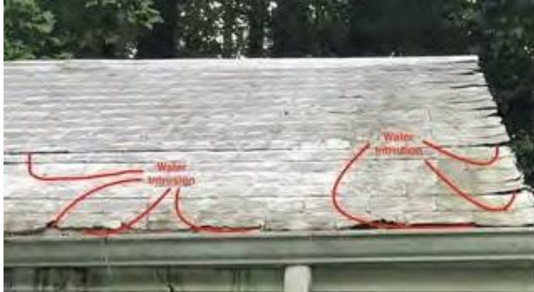
Photograph locations depicted in red where stormwater is intruding the roof of historic Antioch Rosenwald School building interior. Immediate assistance is needed to prevent further damages from the failing roof.
