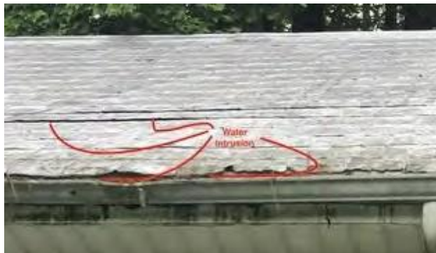
A separate location depicted in red where stormwater is intruding the roof of historic Antioch Rosenwald School building interior. Immediate assistance is needed to prevent further damages from the failing roof.
