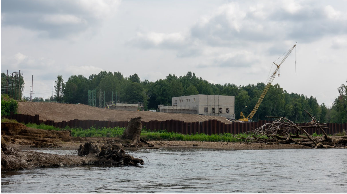
Figure 9: The construction site for the James River Water Authority's water compressor station
