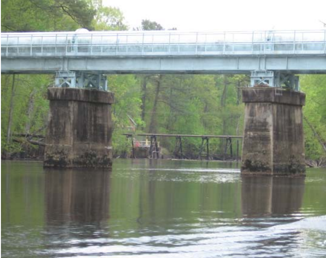
Crossings include road and these pipes
