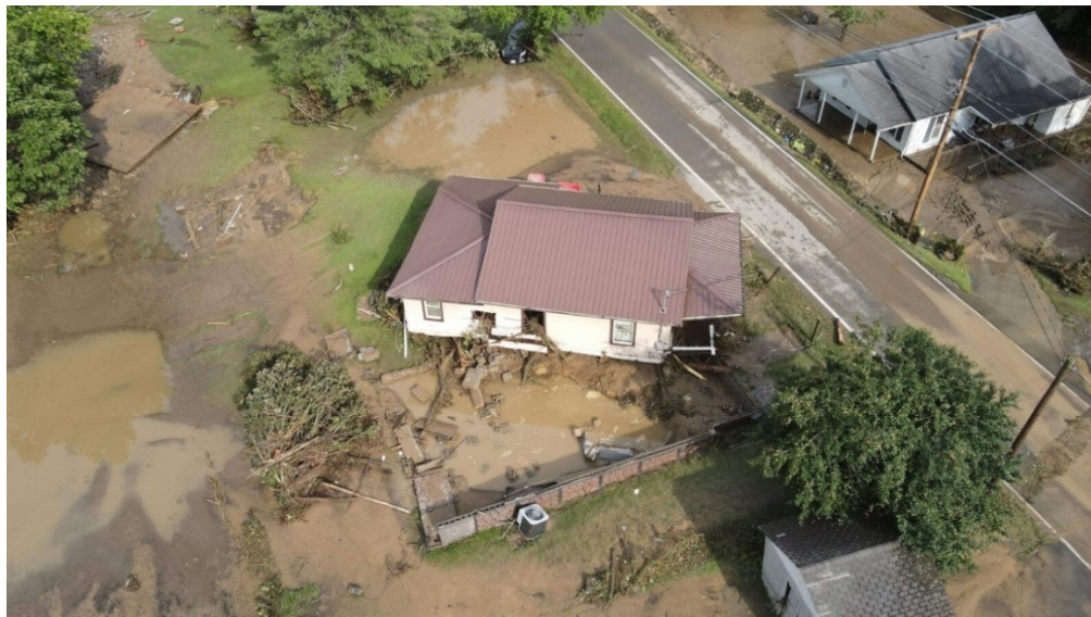
Figure 6-20: Buchanan County home that was pushed off its foundation during July 2022 flooding 36
