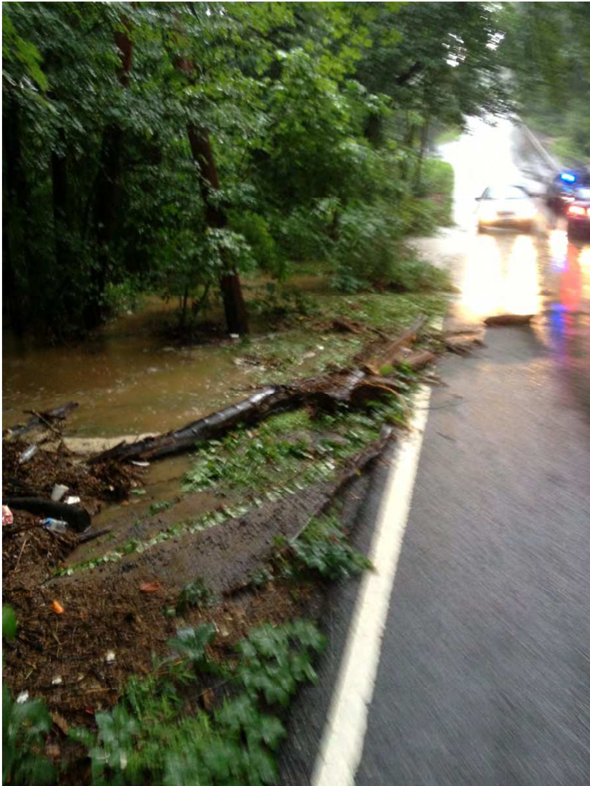
Overtopping at Cherokee Avenue. (taken 2013-06-28)
