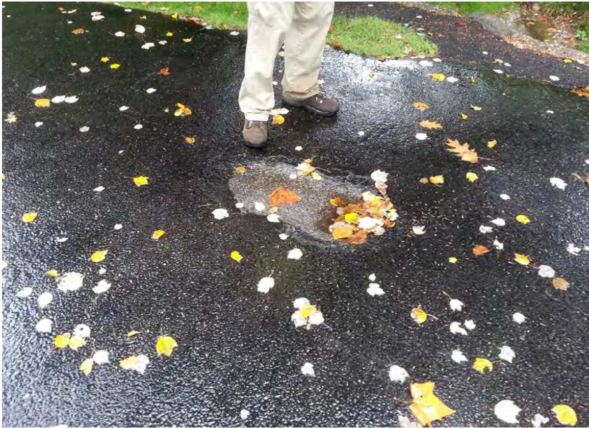
Private property driveway damage
