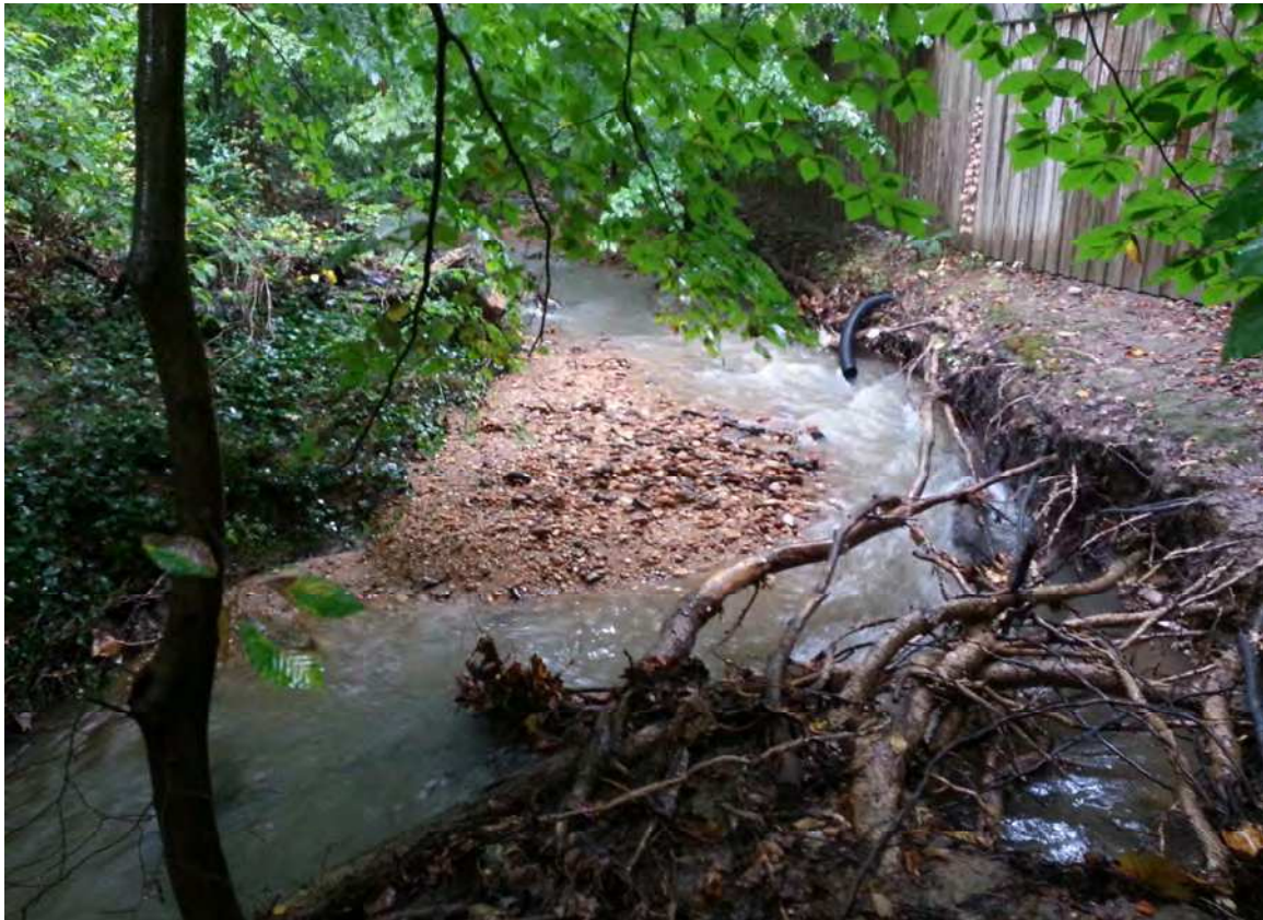
Channel slope erosion
