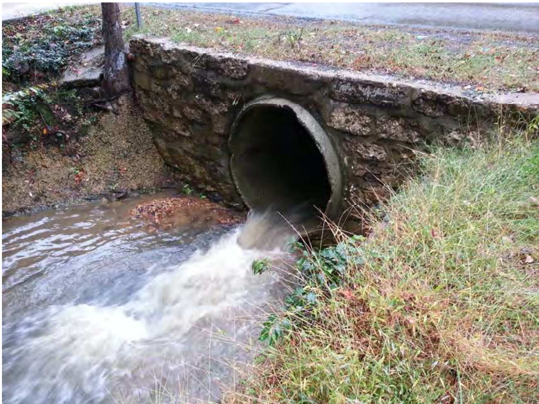
Chowan Avenue crossing outlet.
