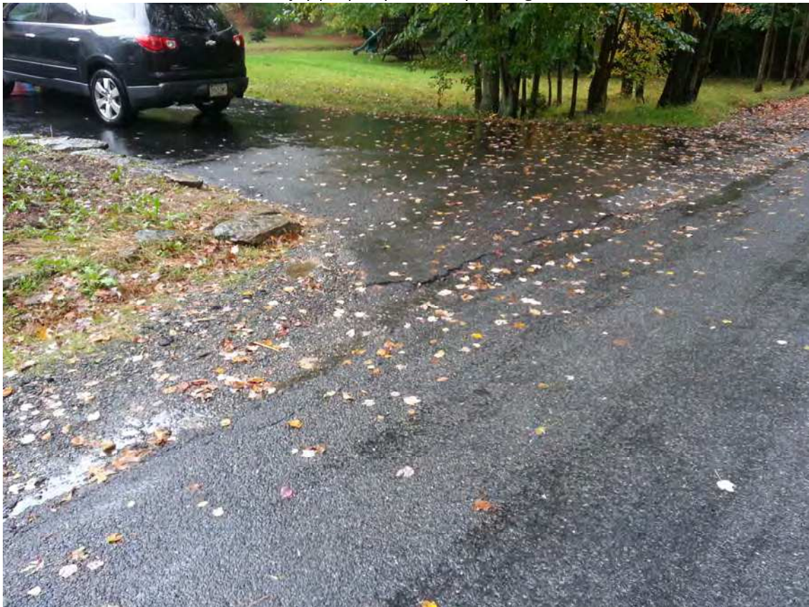
Private property driveway damage
