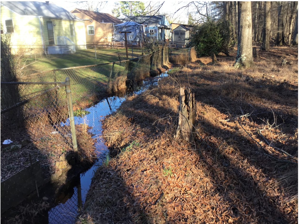
Figure 2. Convergence of Drainage Swales at the Rear of 2012 S. Whitehill Drive.
