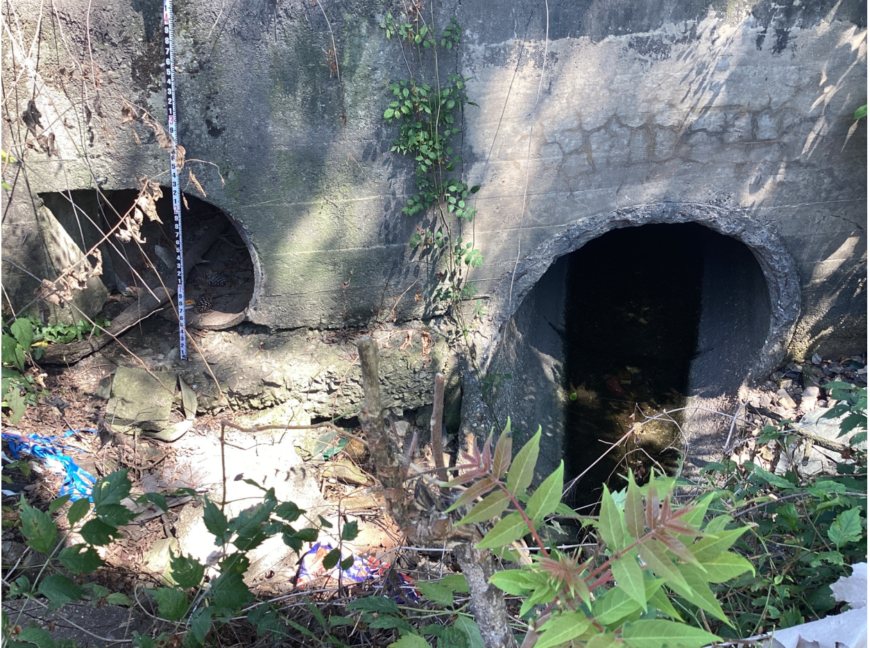
Figure 4. Norfolk and Western Railroad Crossing of Ex. Henrico St Storm Sewer System.
