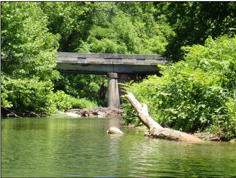
Image 27. Bridge crossing the Pound River. The bridge is Rt. 631/Brush Creek Road.
