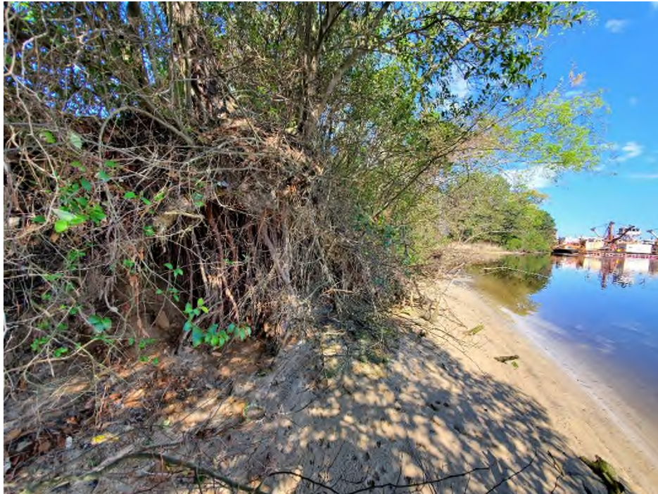
Photo 7: Eroding Bank and Marsh
