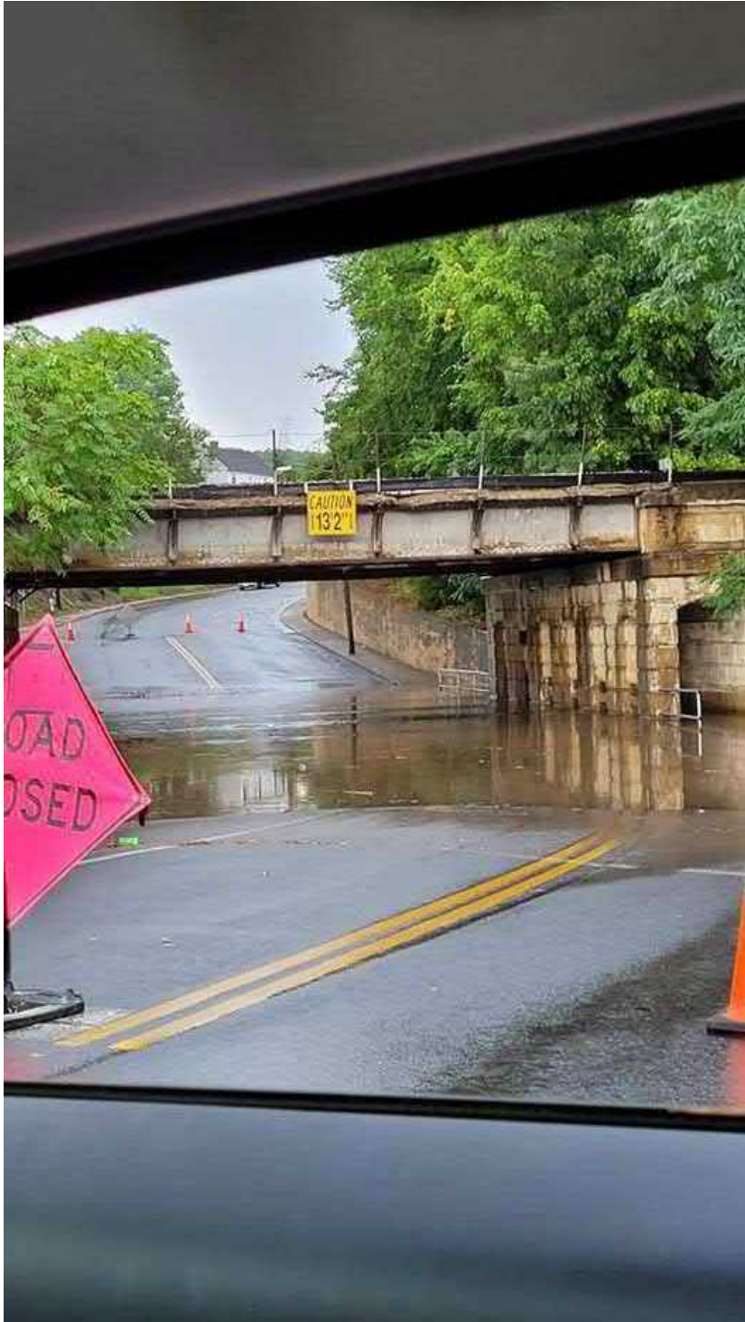
Underpass Flooding (Source: https://www.facebook.com/HighlandsMediaGroup/posts/1209223899532307 )
