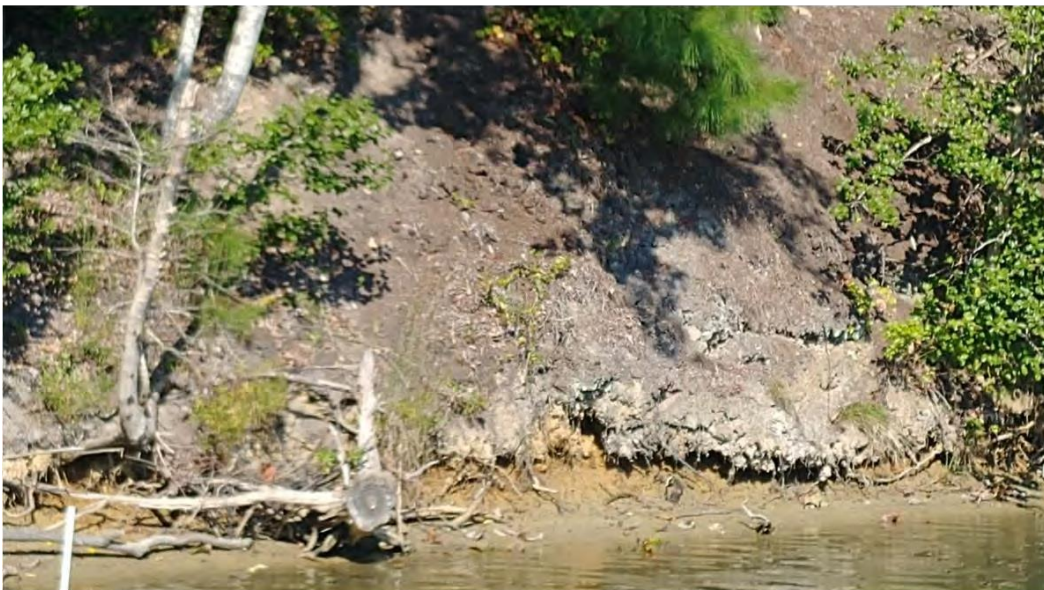
Close-up of the bank erosion on the shoreline. This is where the Envirolok Bags are planned to be installed.
