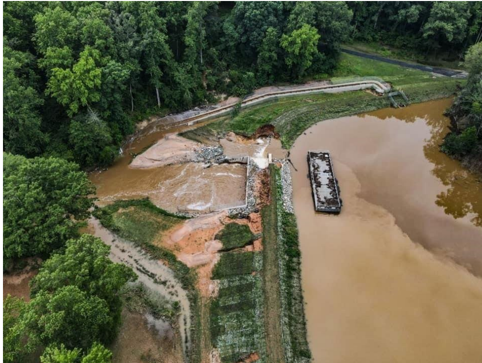
Figure 6-18: Dam Failure at Chandlers Mill Dam
