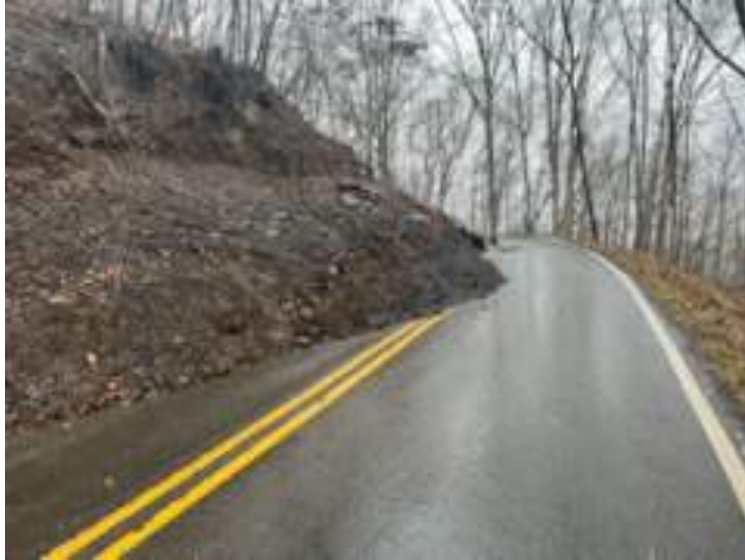
Figure 646: Landslide Event on Route 91, near Tannersville, VA
