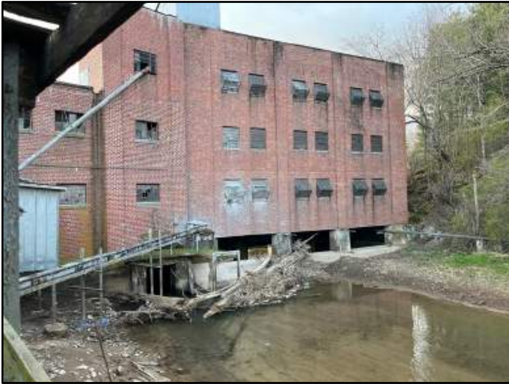
Figure 71: Mill Building March 2023 capturing debris
